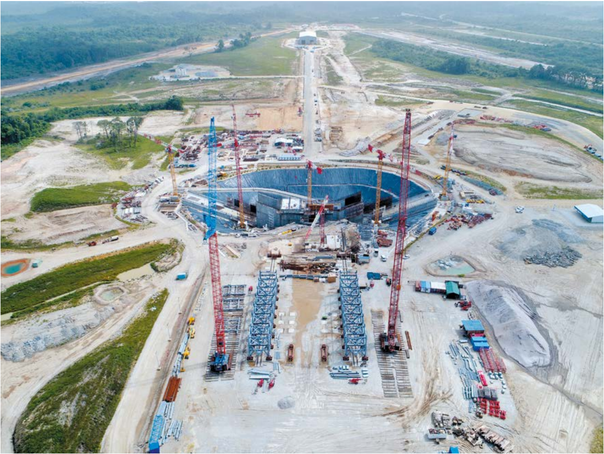
Aerial view of the ELA4 construction site at the Guiana Space Centre.
